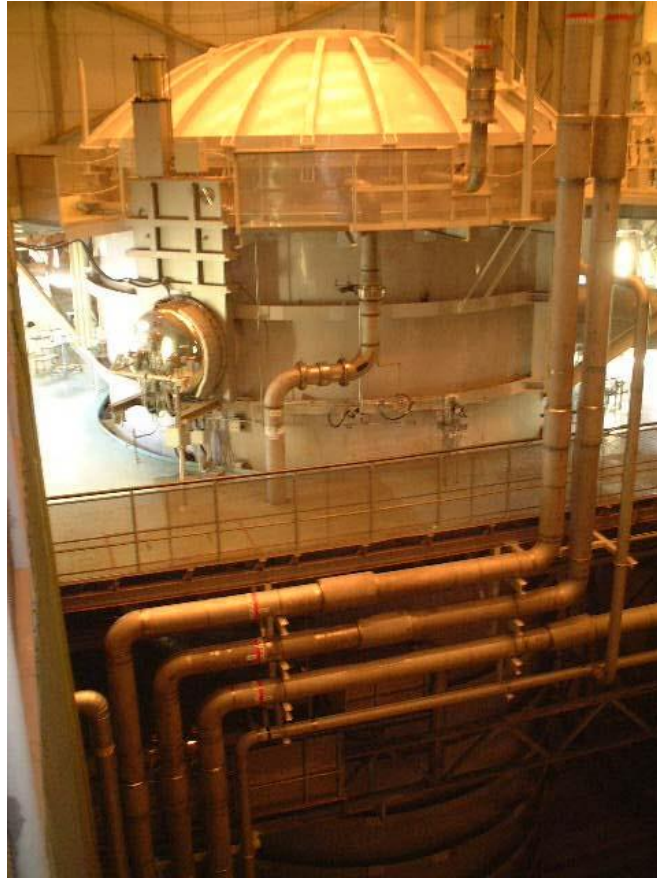
(vacuum vessel/piping system)
